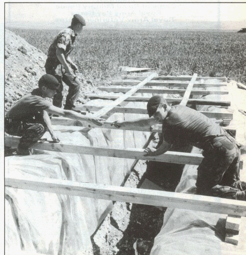
Not the nicest of jobs, but it has to be done. Men of 59 (Independent) Commando Squadron RE construct deep latrine ditches in Iraq
